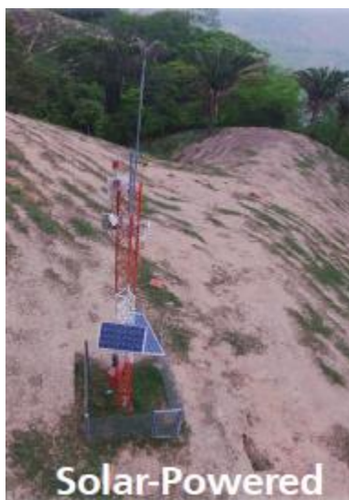
Figure 259 - Solar powered WiBACK node
